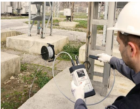
Ground grid continuity testing with RMO-EH
