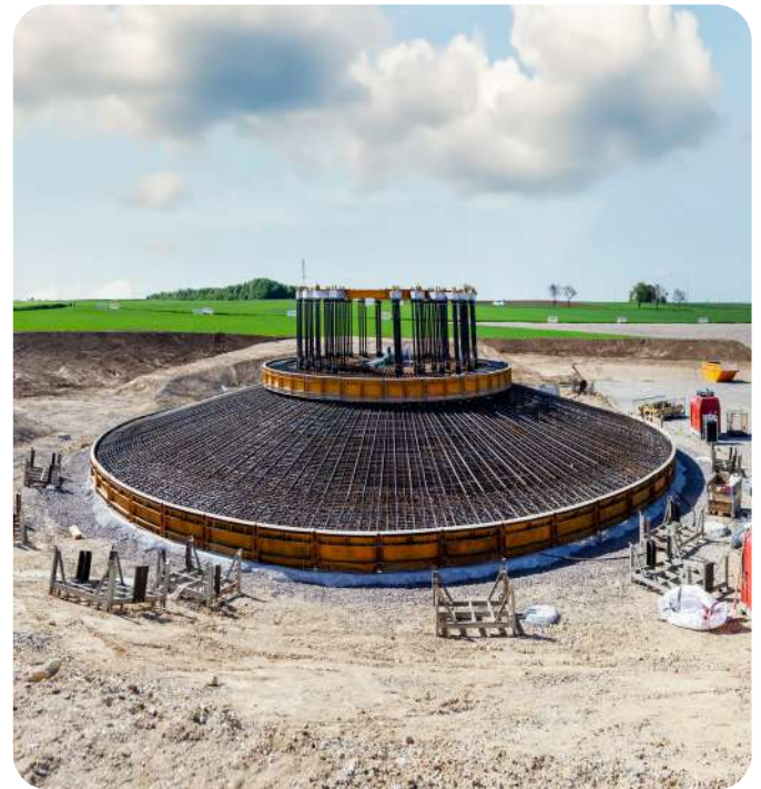
Wind turbine foundation
